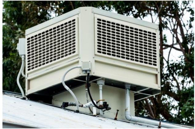
This photo gives you a good insight into the amount of work John Bach has put into the cooler installation.
